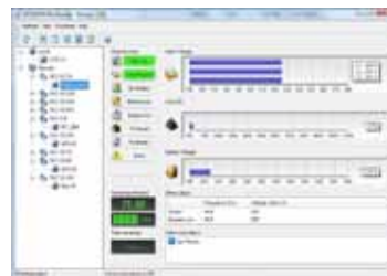
DETAILED UPS PARAMETER DISPLAY PowerShield 3 provides all the information required for first level diagnostics.
